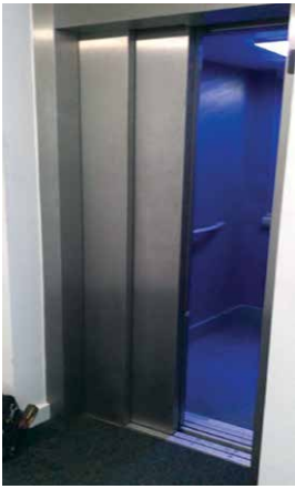
Figure 1: Image of landing and lift car doors showing measurement positions
