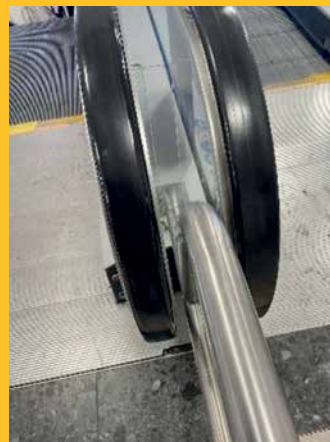
Luggage barrier too close to escalator handrail presenting trapping hazard
