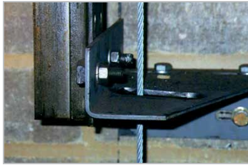
Figure 3 Incorrectly installed governor rope
